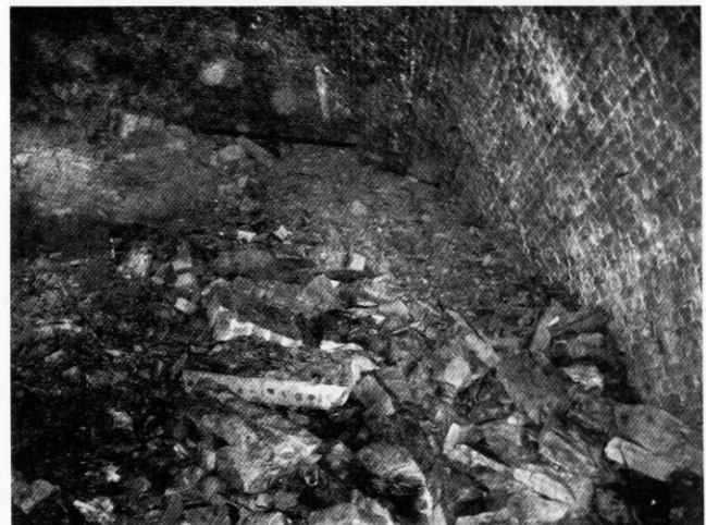
Roof collapse at the far end of the tunnel. Only 80m of tunnel is now accessible. Photo by Peter Jigins
